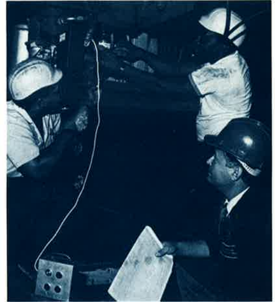
Installing a new Knorr Air Compressor (left to right) Ronald Ford, CME; Cecil Clarke, CME; and Leon Sanevich, Maintenance Supervisor II.
