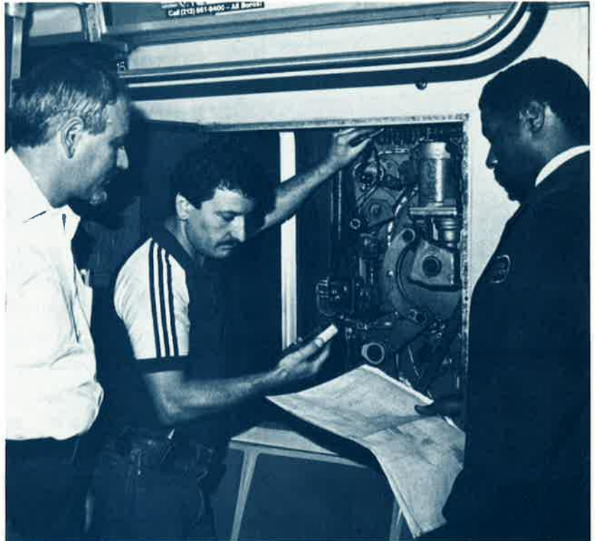
Checking door control circuit voltages (left to right) Salvatore Scarpaci, Maintenance Supervisor II; Mike Belloli, CME; and Russ Woodley, AET II.
