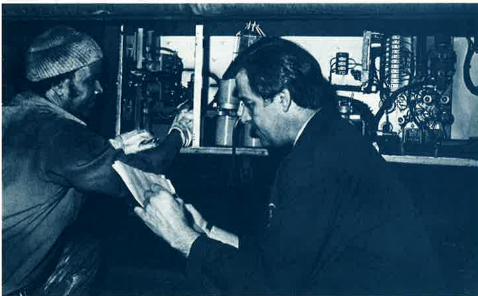
Replacing a defective SCR (Silicon Control Rectifier) (left) Homer Lawrence, Car Inspector and Jerry Gottehrer, Project Manager (right).
